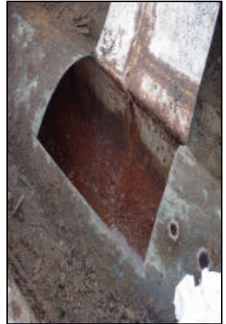
Picture of an unregulated heating oil tank
